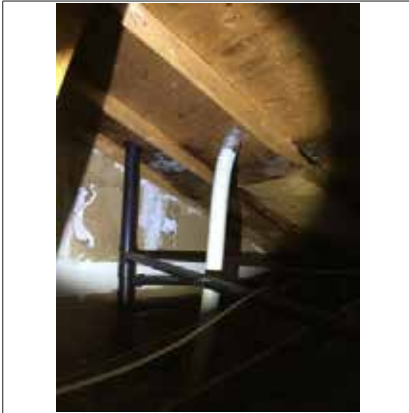
Sheathing discoloration and stained
