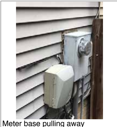
Meter base pulling away
